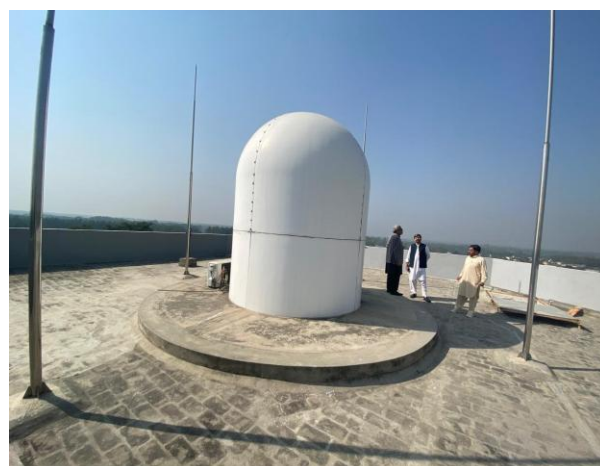
Photo 14: X-band Weather Surveillance Radar at the Flood Forecasting and Warning System, Fazal Abad, Mardan, observed during the field visit and focus group discussion with FFWS staff on 24 October 2025.
