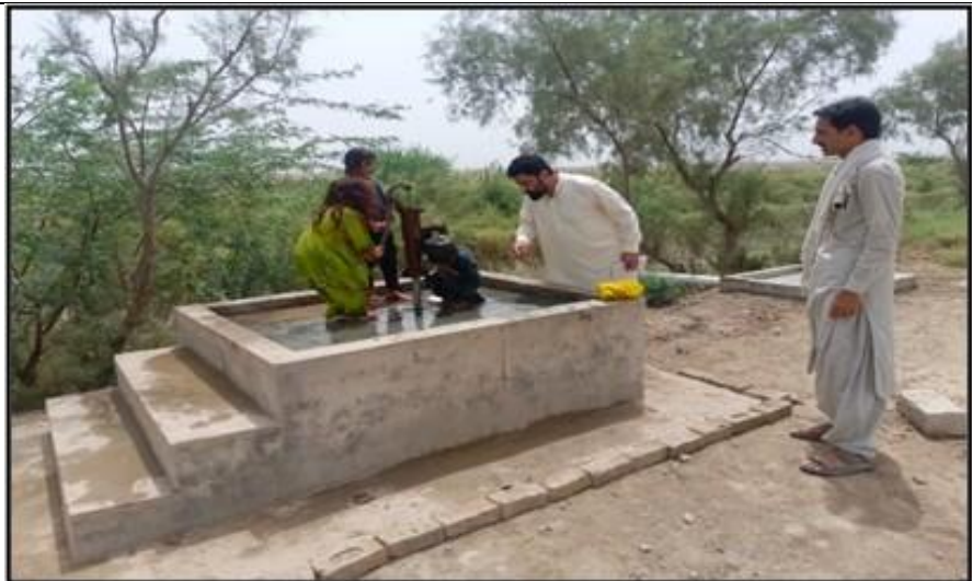
Handpump with washing pad
